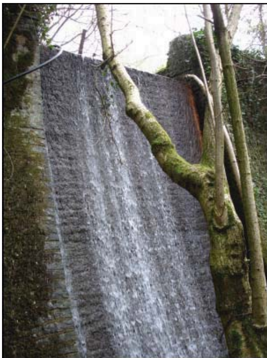
The Benson Brook Hydro Dam
