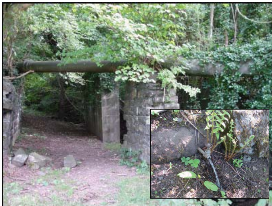
Penstock crossing the brook at Bitterley Junction and inset water still flowing
