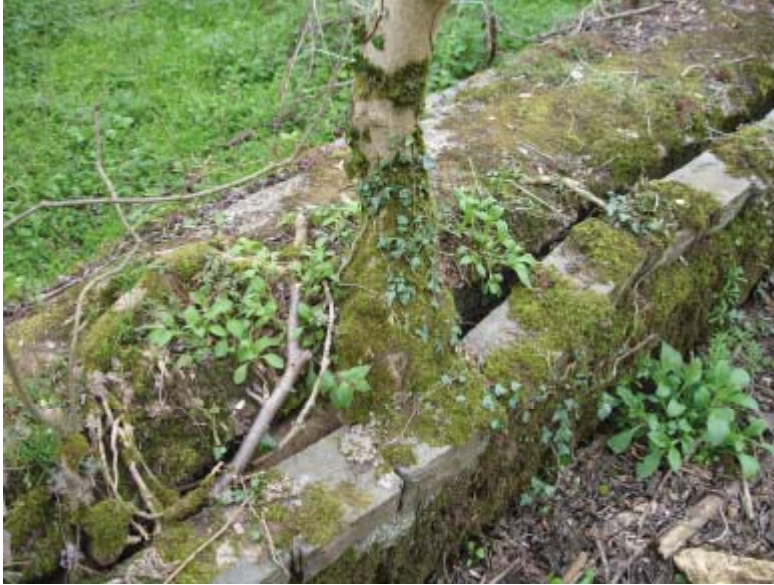
Tree damage to dam wall
