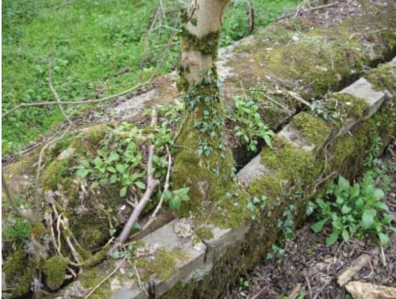
Tree damage to dam wall
